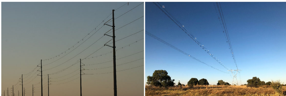
Figure 2. Powerlines marked with BFDs in Namibia. Left: flappers alternating with spirals on each earth wire of two powerlines running parallel to each other. Right: White spirals along one earth wire and black spirals along the other earth wire on a 400 kV transmission powerline, northern Namibia (photos: J. Pallett).
